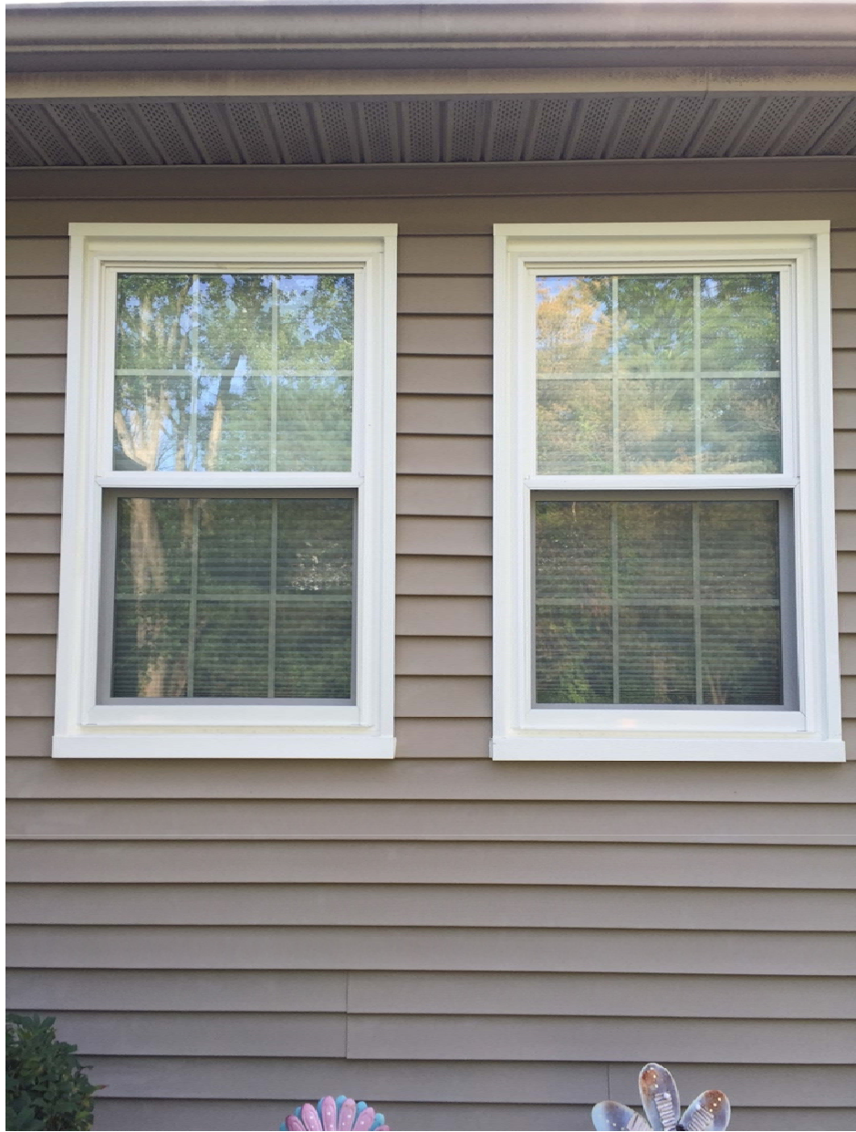
Incorrect Window. Over the "J" Channel
