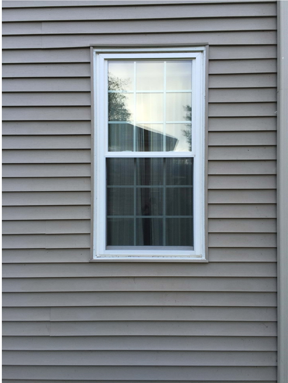
Correct Window. "J" Channel exposed.
